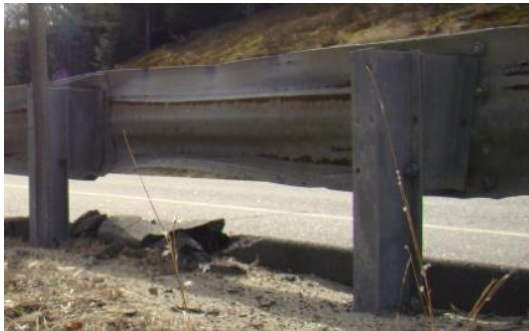
Field Example of Rail Flattening
