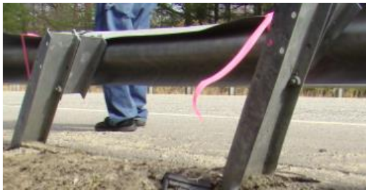
Field Example of Rail Crush
